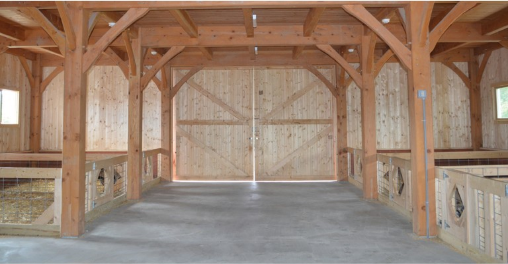
▲ The owner's preference for a lack of visible fire suppression materials in an exposed structural frame led to the selection of the heavy timbers shown here in the first floor. Photo Courtesy of A.R. Brouwer Company
